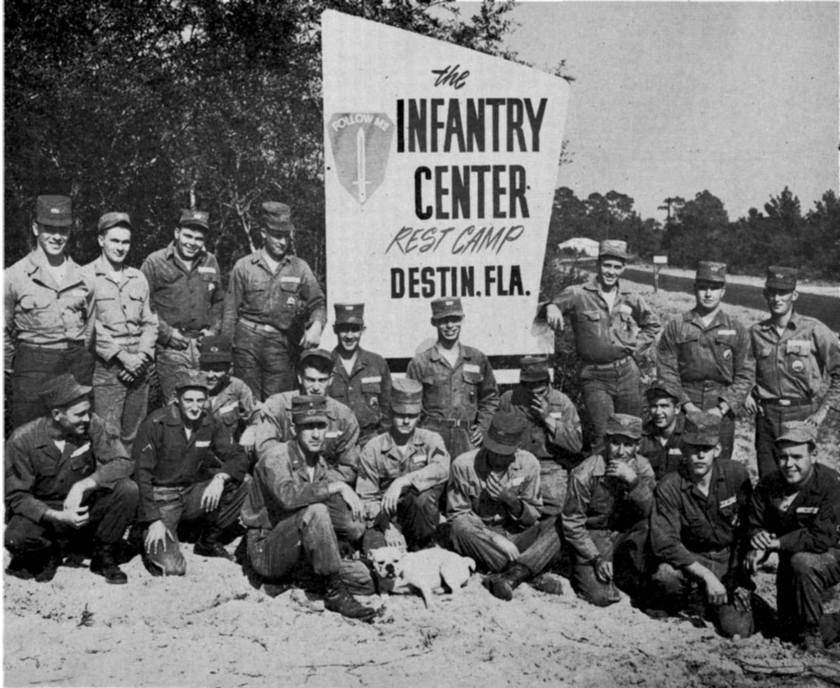
LAST SEPTEMBER THE ENGINEERS OF THE 508TH ABN RCT WENT TO DESTIN, FLORIDA TO GIVE A FACE LIFTING TO THE TIC REST CAMP LOCATED THERE. THEY TURNED A RUN-DOWN AREA INTO ONE OF THE FINEST VACATION SPOTS ON THE FLORIDA COAST.
