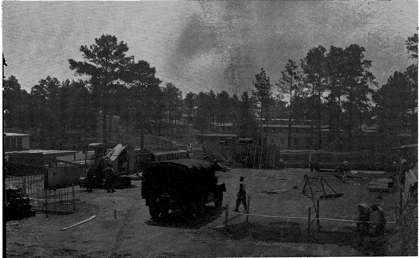
THE 78TH ENGINEER BATTALION WORKS ON MAJOR PROJECTS FOR THE POST. HERE THEY CONSTRUCT THE SWIMMING POOL AT HARMONY CHURCH.
