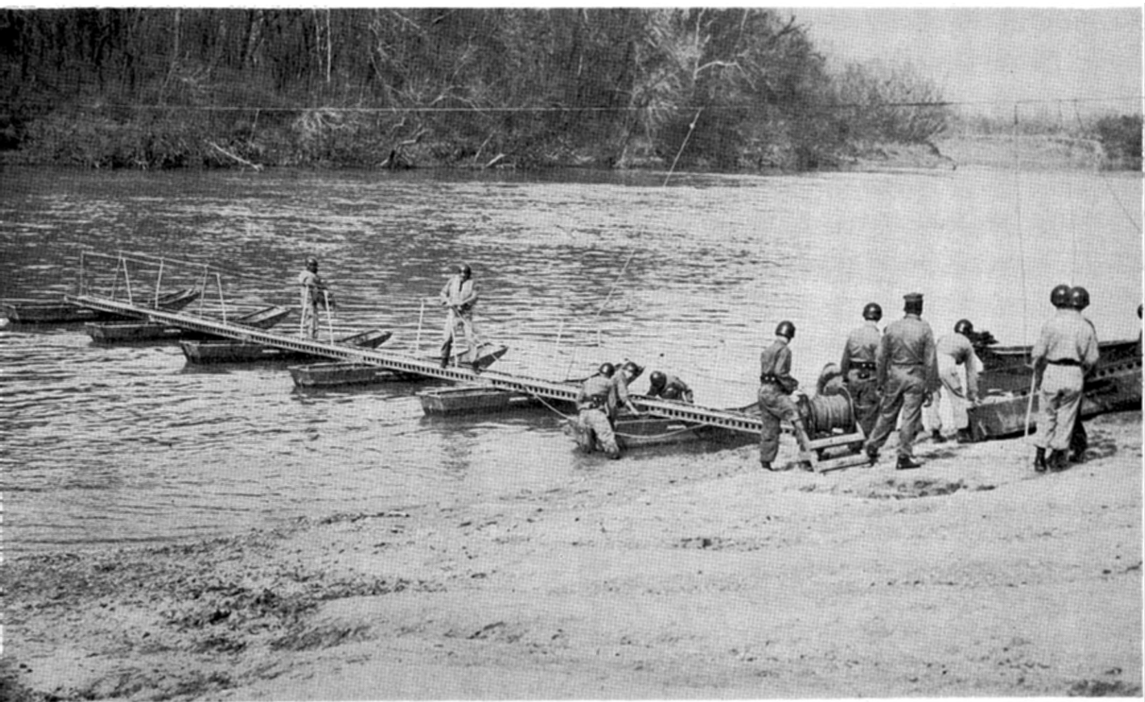
PARTING THE WATERS ENGINEER STYLE. THIS FOOT BRIDGE CAN BE THROWN ACROSS THE CHATTAHOOCHEE RIVER IN SIX MINUTES
